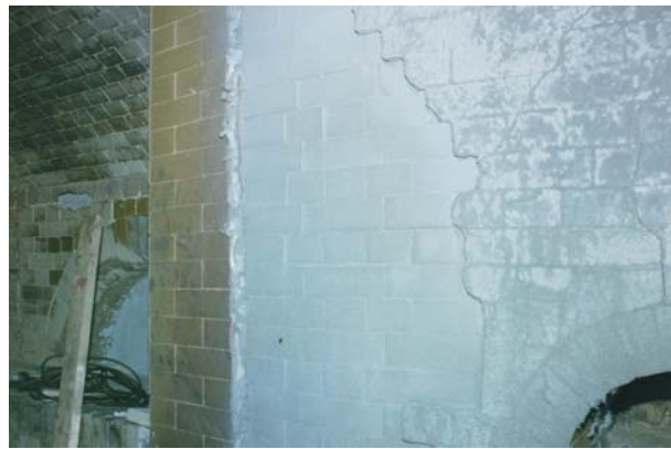
Fig. 7: Tunnel kiln preheat section (right 2/3 of photo) after application of high emissivity coating. The textural differences between the new and used refractory brick surfaces are obvious.
